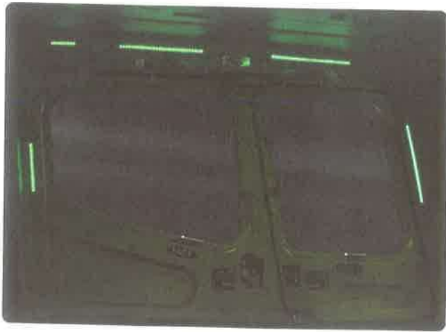
Figure 9-24. Emergency egress lighting in a medium size helicopter.
