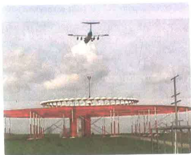
Figure 7-114. A VOR with DME ground station.
