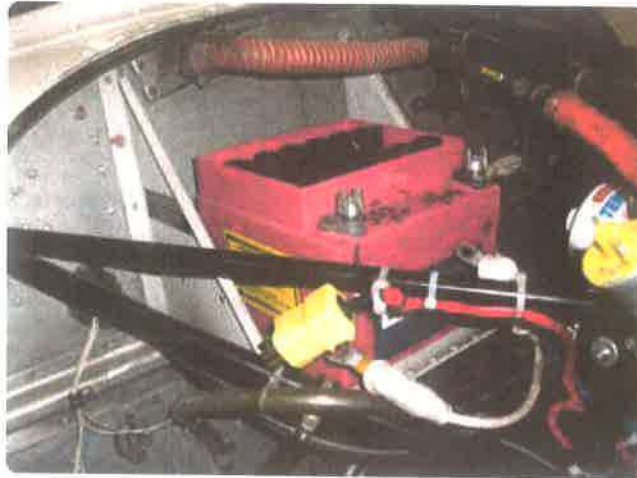
Figure 8-2. Lead acid battery installation.
