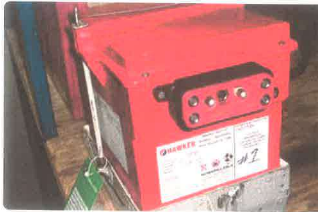
Figure 8-3. Valve-regulated lead-acid battery.
