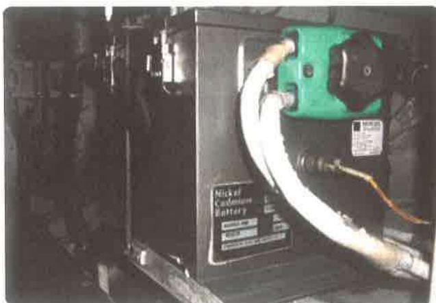
Figure 8-4. NiCd battery installation.
