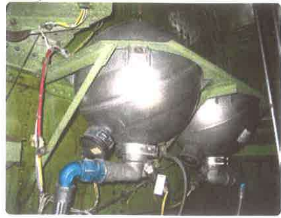
Figure 10-11. Built-in non-portable fire extinguisher containers (HRD bottle).
